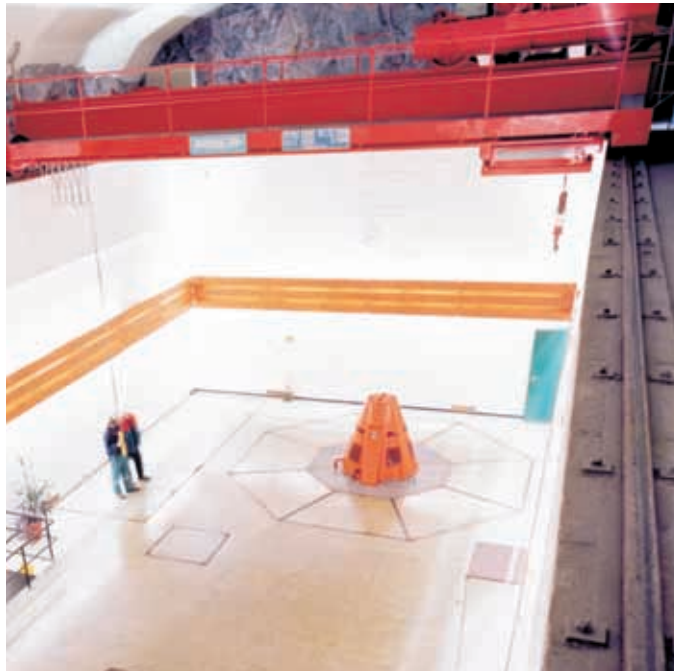
Elkem's power plant at Bremanger.
