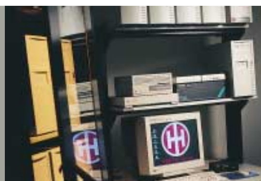
Equipment to simplify and make the server room more efficient.
