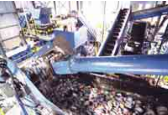
TOMRA processing facility in Quebec, Canada. Photo: TOMRA.
