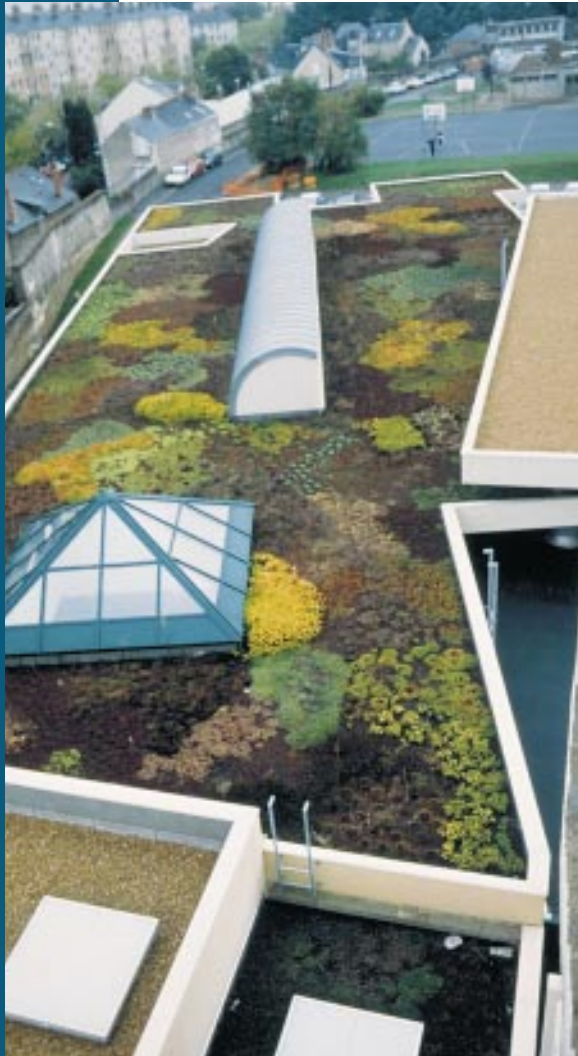
The green terrace at this school in Angers, France, has 20,000 plants. Siplast's roofing system was chosen on aesthetic, ecological and acoustical grounds.
