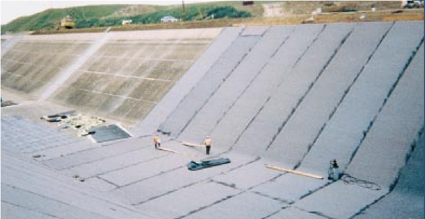
More than one million square feet of Siplast Teranap geomembrane were used to repair the California Aqueduct.
