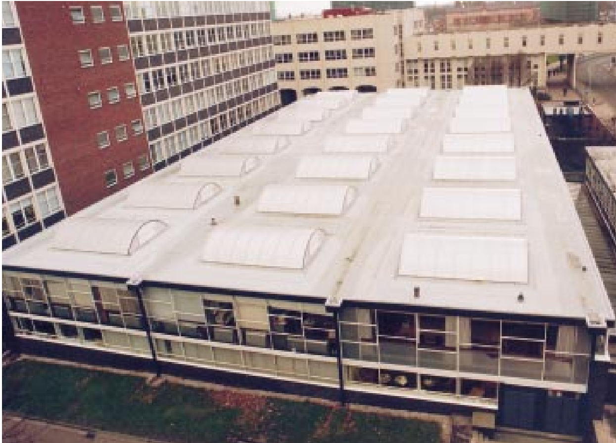
This renovation work at Manchester University involved the replacement of 1,600 m 2 of flat roofing. The Anderson Profile system, which consists of a vapour barrier, insulation, underlay and top felt, was used.
