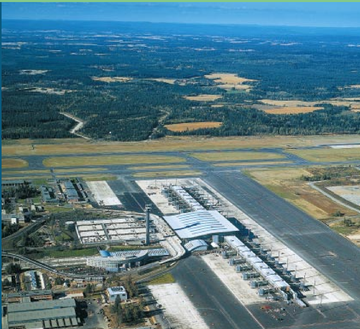
Icopal has carried out roofing on the new airport, Gardermoen, in Norway.
