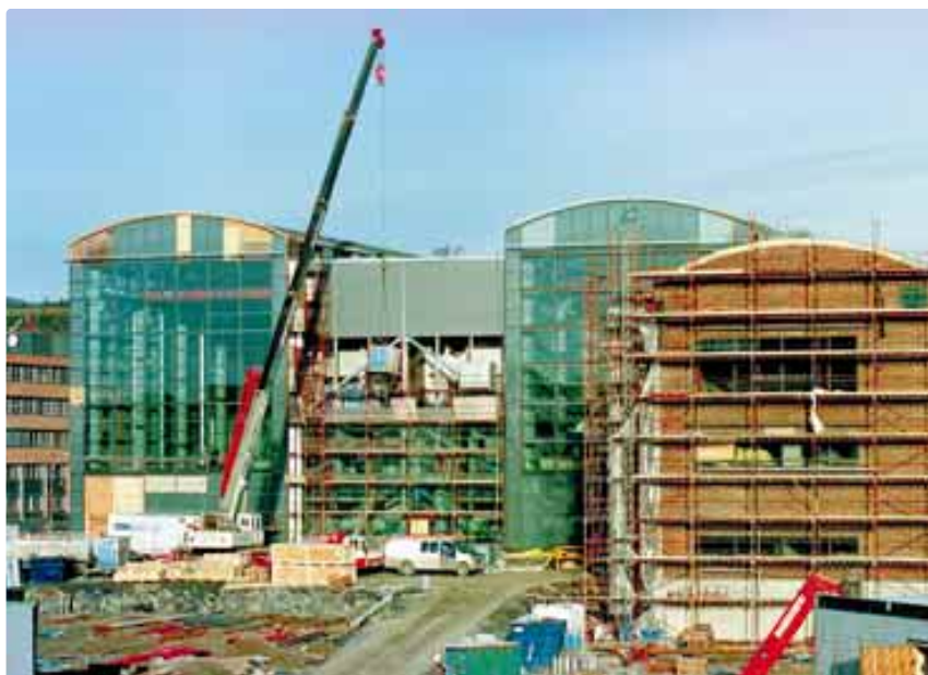
The new printing plant at Nydalen in Oslo will cover an area of 41,000 square meters and will have capacity to produce 4.5 million newspapers per week.
