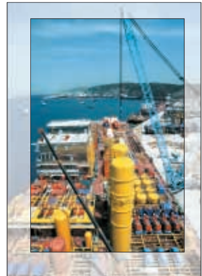
GIRASSOL FPSO PROCESS EQUIPMENT
