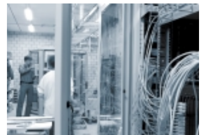
The new server center.
