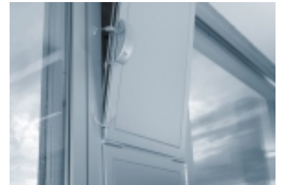
More than 550 FLS were built into the new Belimo wing in Hinwil / Switzerland.
